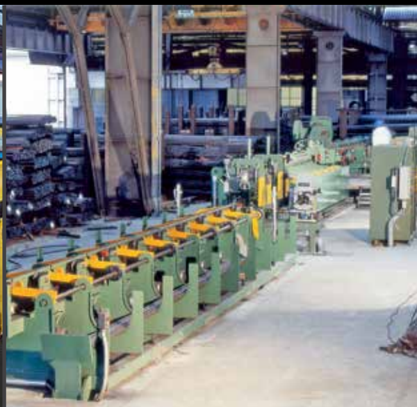
Straightening and Controls
